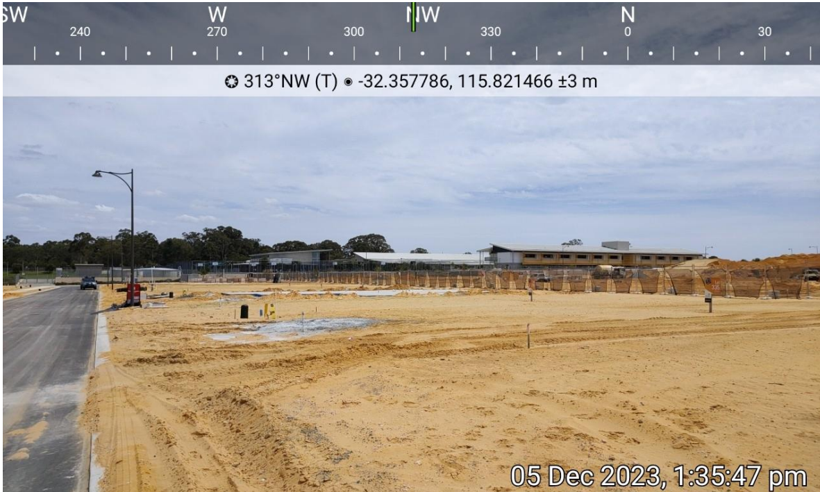
Plate 4: Evidence of external area to lots affected by Condition 9 being cleared and maintained to low threat.
