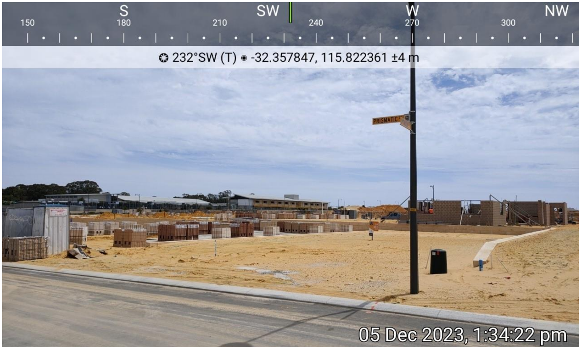
Plate 3: Evidence of external area to lots affected by Condition 9 being cleared and maintained to low threat.
