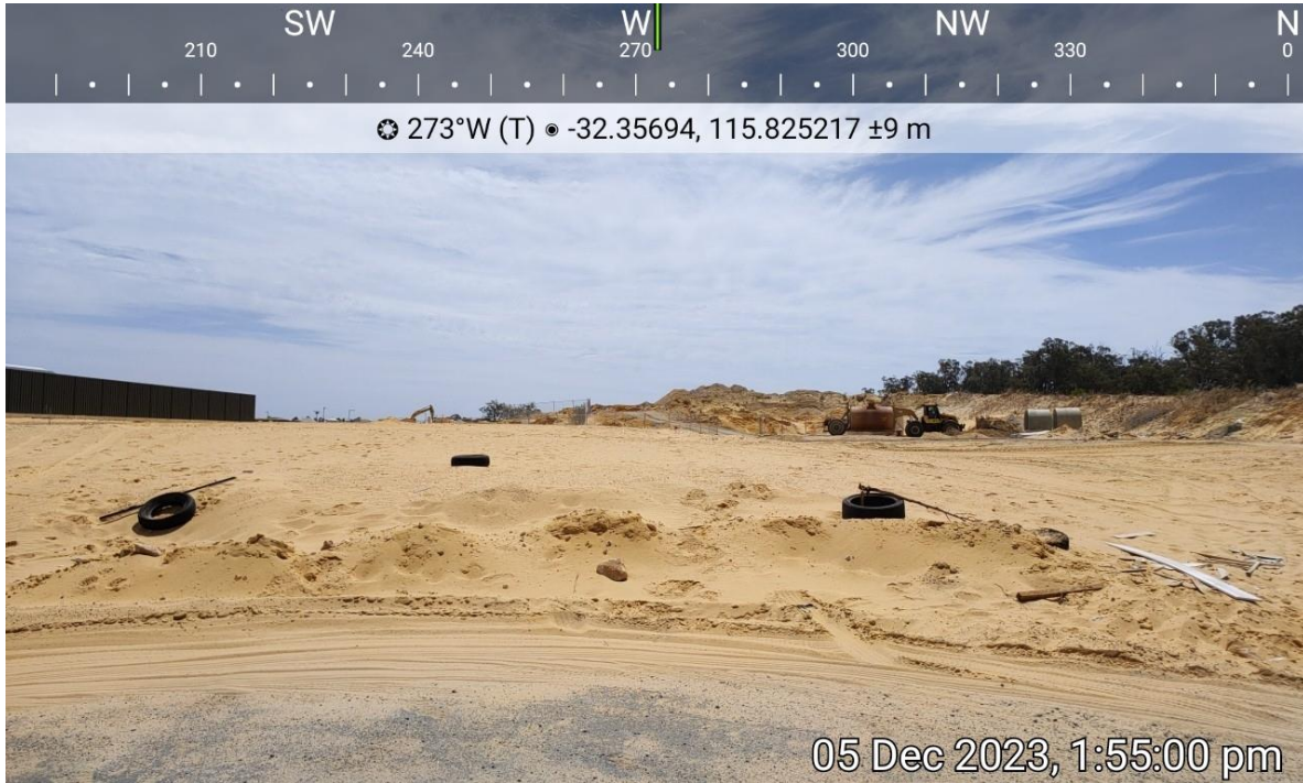
Plate 6: Evidence of external area to lots affected by Condition 9 being cleared and maintained to low threat.
