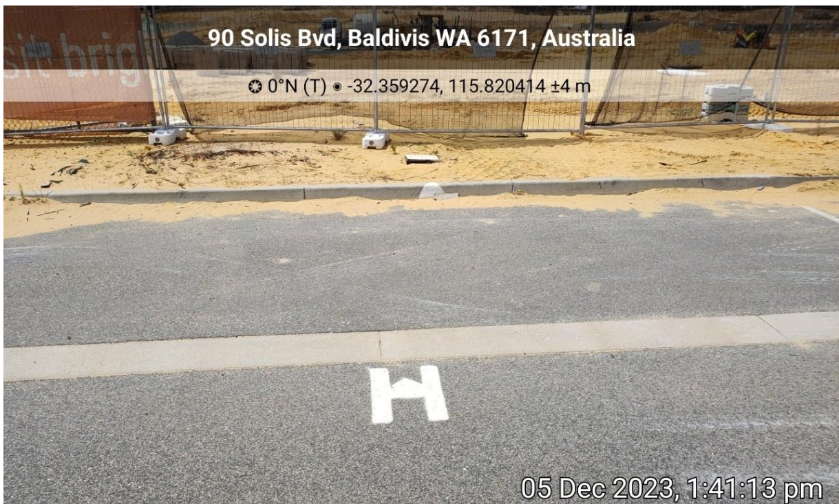
Plate 10: Evidence of external hydrants present in surrounding area.
