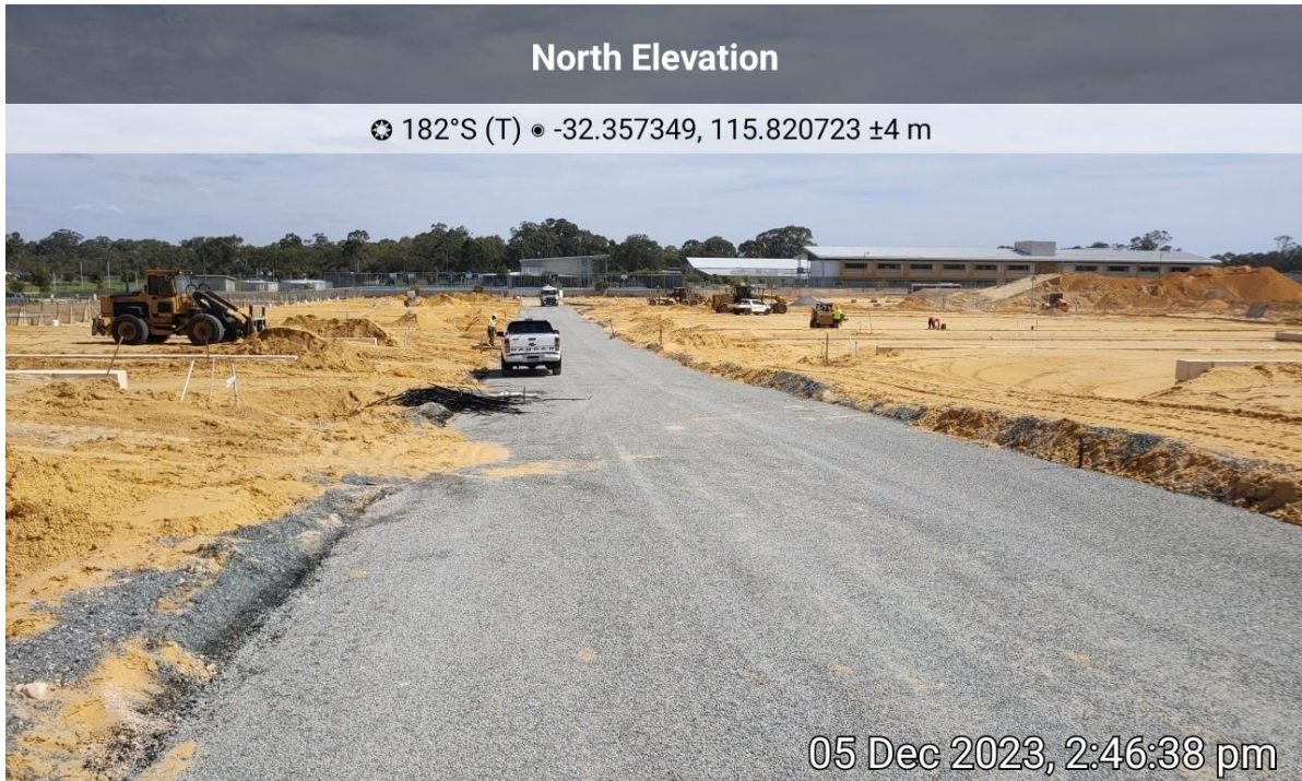
Plate 5: Evidence of construction of internal roads is underway in accordance with Roadworks Layout Plan.
