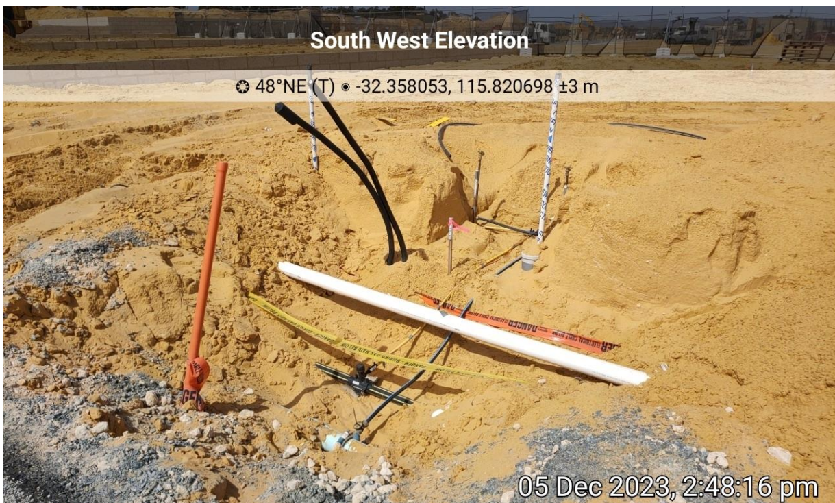
Plate 8: Evidence of installation of reticulated water within construction site is underway in accordance with the Water Reticulation Plan.
