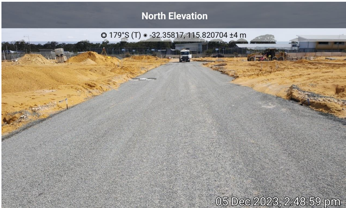
Plate 6: Evidence of construction of internal roads is underway in accordance with Roadworks Layout Plan.
