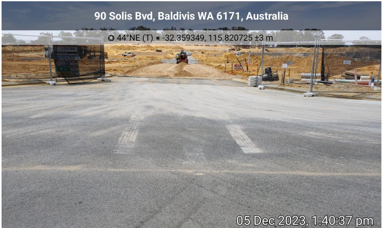
Plate 7: Evidence of construction of internal road connection to external road network is underway in accordance with Roadworks Layout Plan.
